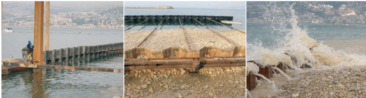
Installation of waling at retaining wall before actual quay wall construction will start.
